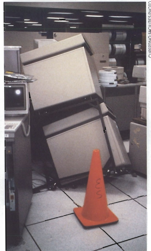
In Cupertino, seismic force slid this disk-drive rack into a floor opening.
